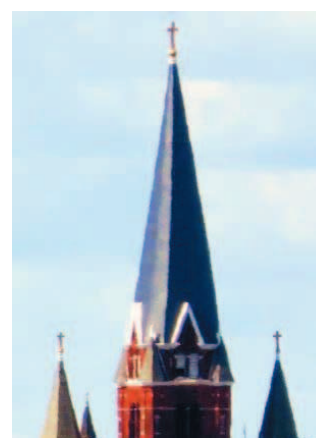
Newly repaired and restored St. Josaphat Church Steeple (as seen from Detroit Tigers' baseball stadium). A beacon for more than a century.
