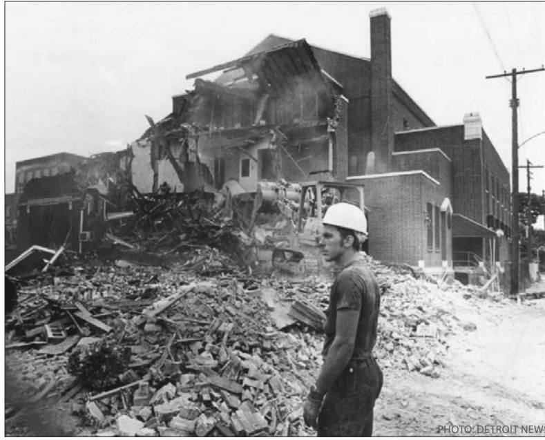
Poletown's Immaculate Conception Church under the wrecker's ball, July 15, 1981. General Motors and the cities of Detroit and Hamtramck relied on eminent domain to relocate the 4,200 people who lived in the area — including their 1,300 homes, 140 businesses, six churches and one hospital — to build an automobile plant. Last month, GM announced the closing of the plant.
